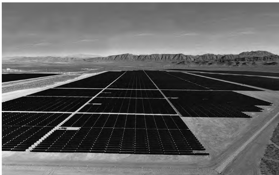
250-megawatt Beacon Solar Plant located in the Mojave Desert near Cantil, California
